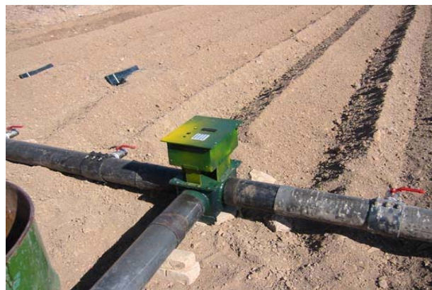
Fig. 2. Controller of the butterfly valve
